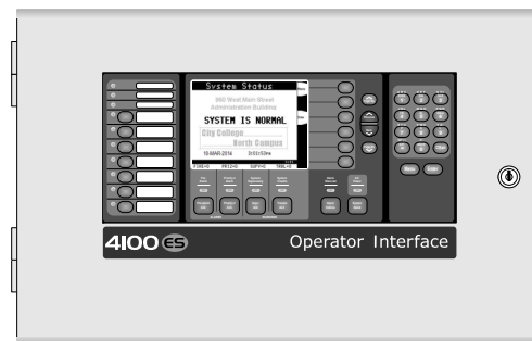
InfoAlarm Command Center in Remote Cabinet
