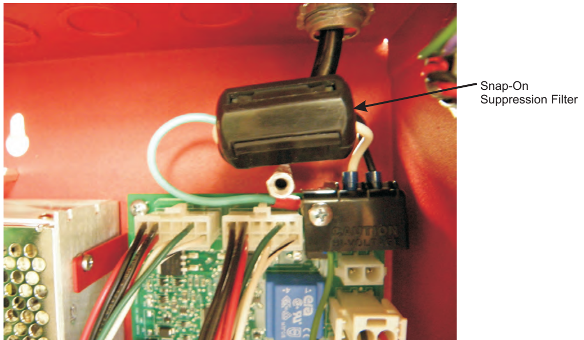
Figure 2-10. Snap-On Suppression Filter Shown Installed Around Black and White AC Power Wires
